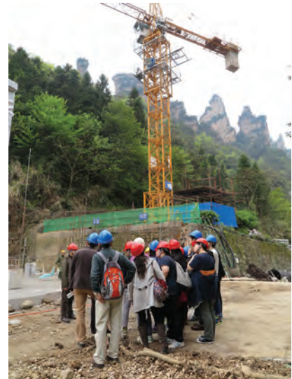
Chu Hai students visit the construction site of the redevelopment of the cableway.
